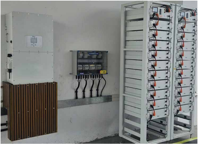
India ▶ Inverter: SUN-50K-SG Capacity: 50kW
