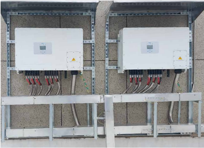
China ▶ Inverter: SUN-110K-G Capacity: 220kW
