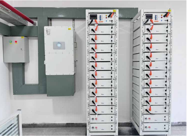
China ▶ Inverter: SUN-50K-SG01HP3-EU Battery: BOS-G Capacity: 50kW/100kWh
