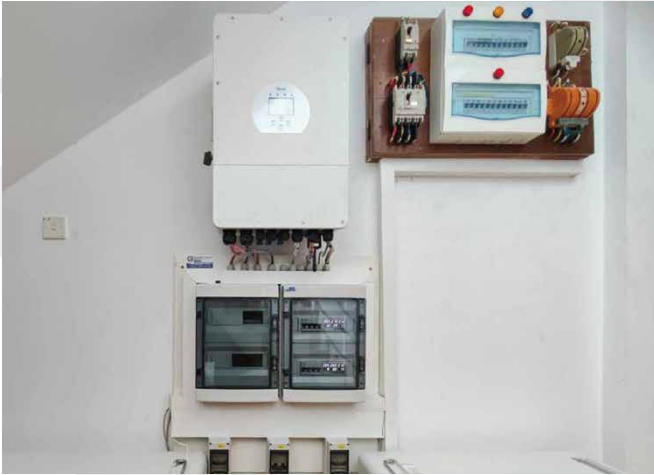
Myanmar ▶ Inverter: SUN-12K-SG Capacity: 12kW
