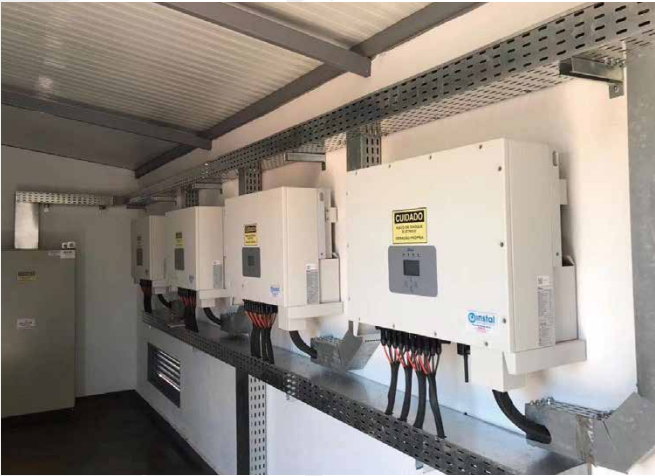
Brazil ▶ Inverter: SUN-80K-G Capacity: 320kW
