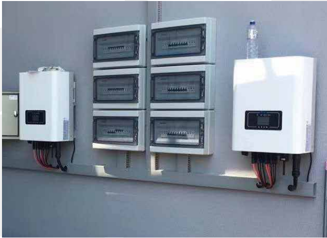
Brazil ▶ Inverter: SUN-25K-G Capacity: 50kW
