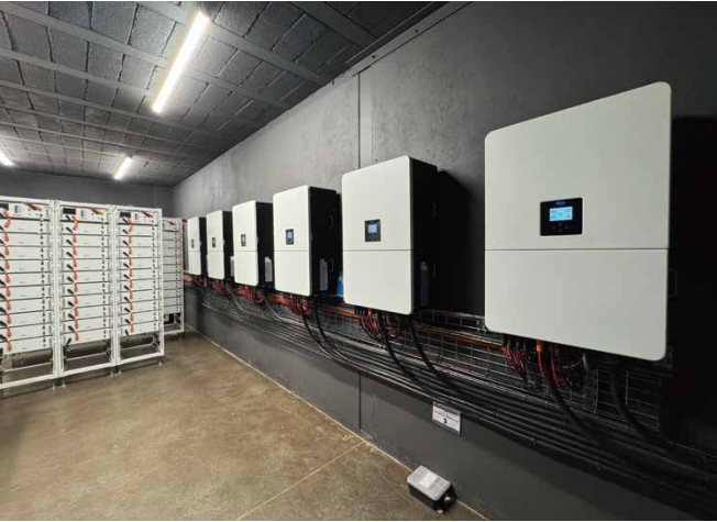
Zimbabwe ▶ Inverter: SUN-80K-SG02HP3 Battery: BOS-G/BOS-G Pro Capacity: 480kW/660kWh
